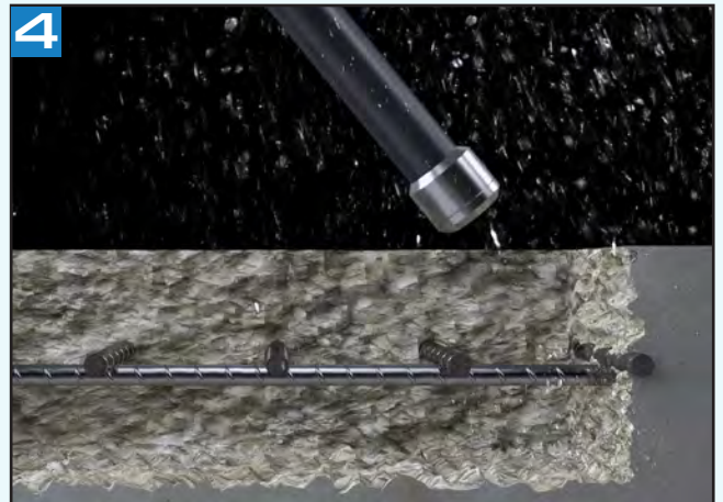
The remaining area consists of structurally sound concrete and is now prepared for the application of a new layer.
