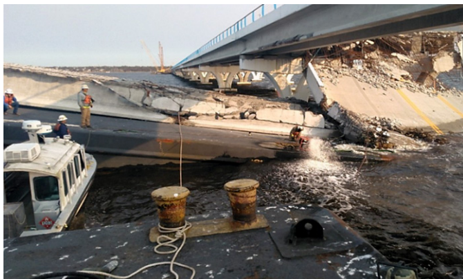
Seven spans of the Pensacola Bay Bridge required either partial or full replacement after suffering devastating damage from loose barges during Hurricane Sally.
